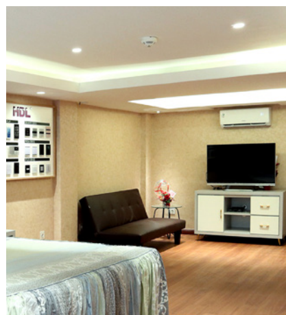
Putra Makmur Abadi, Medan Lighting, AC & Curtain control
